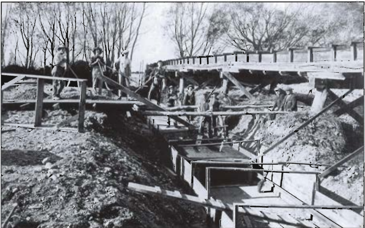
Construction of the syphon under the Eyre River at Wolffs Road. The builders were George Smith and Son of Oxford. May 1913.
