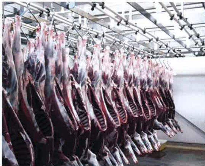
Carcass moved to chiller and spray chill system The spray chill system minimises weight loss whilst the carcass is in the chiller and decreasing the time taken to reach optimum chill temperature of 4 °c for boning.
