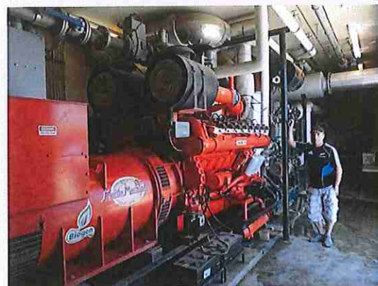
FIGURE 3- IN CALIFORNIA, A DAIRY FARMER IS PRODUCING METHAN GAS FROM EFFLUENT AND SELLING ELECTRICITY TO THE GRID
