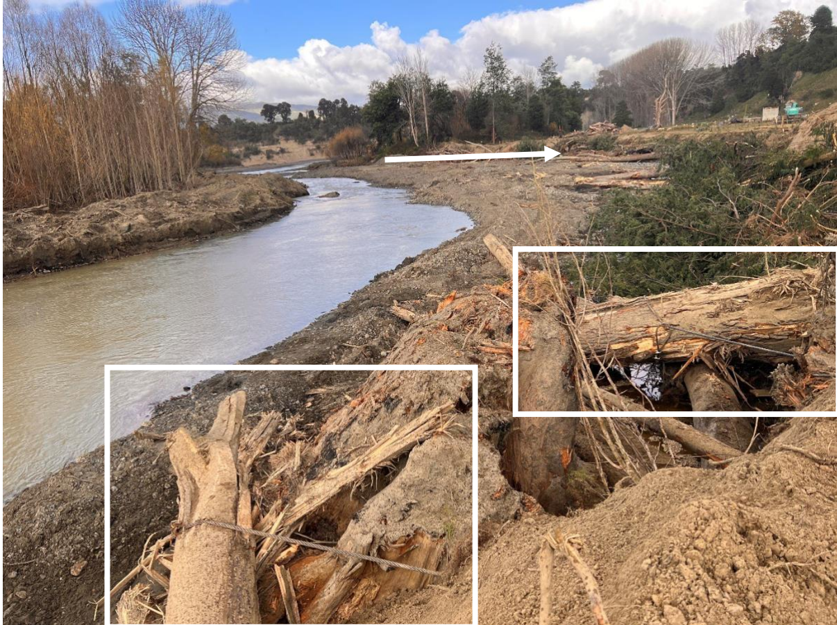
Figure 9 This creek flooded during Cyclone Gabrielle, causing erosion to the riverbank and threatening close-by infrastructure. As can be shown in the two boxes and arrow, a groyne is under construction to mitigate future loss on this property.
